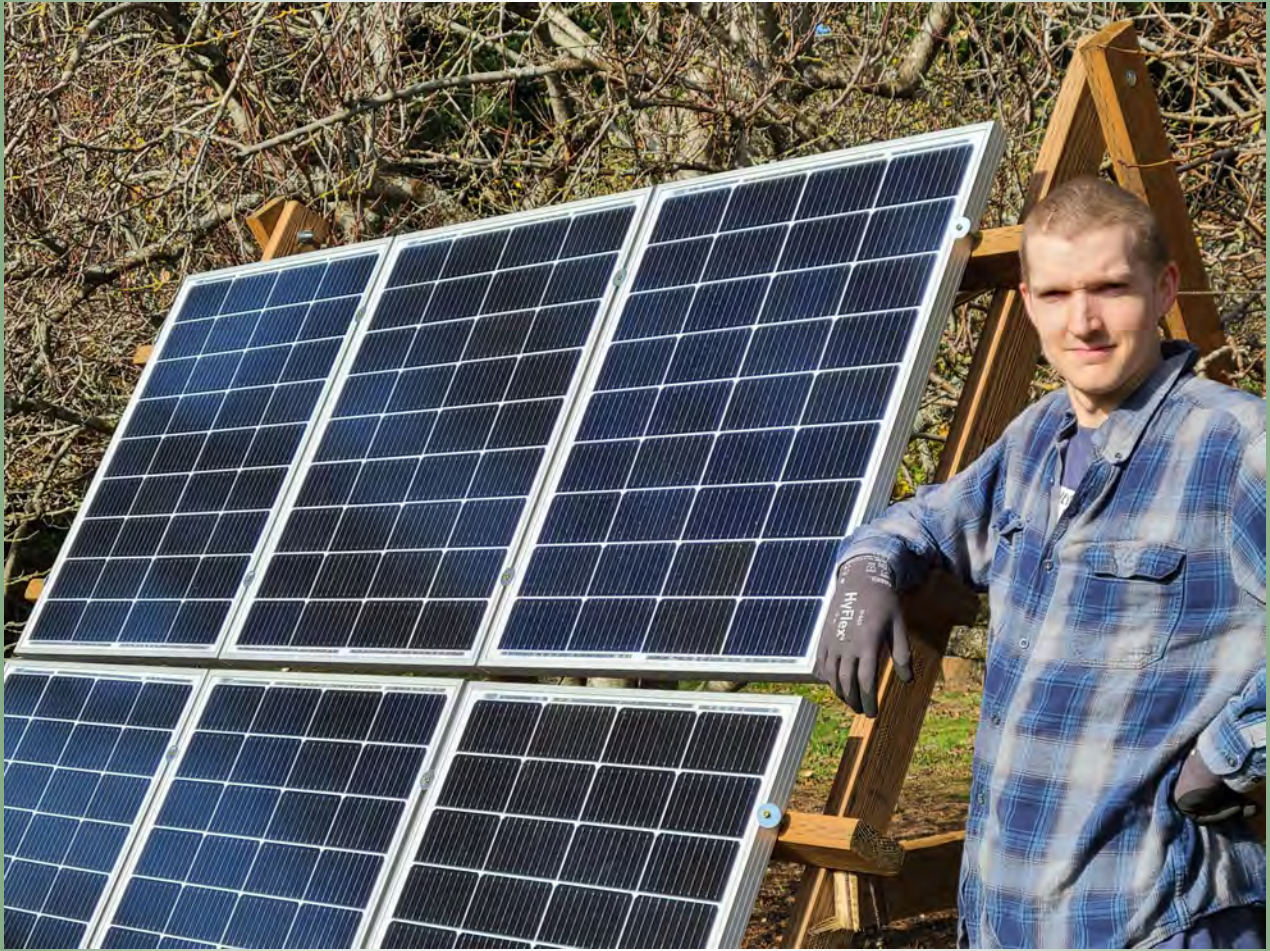
Donovan Clark of WISS with the solar array portion of the solar power system he built.
